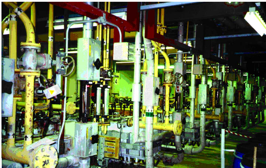
Figure 12. Modern fluorine generation. The fluorine cell room used in the manufacture of per-fluorocarbon gases and fluids, F2 Chemicals Ltd, Preston, UK. (Photograph: M. Atherton, F2 Chemicals Ltd.)
